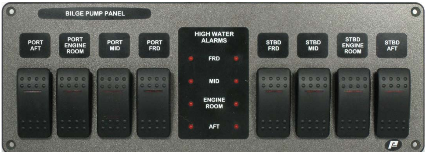
RA110A has an embedded high water alarm panel
